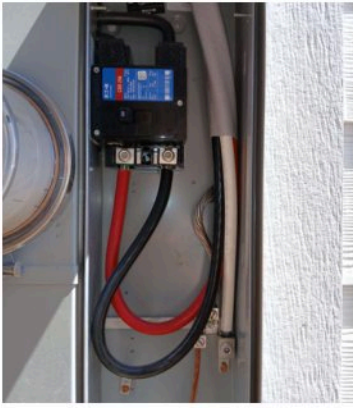
Main disconnect interior showing neutral-ground bonding
