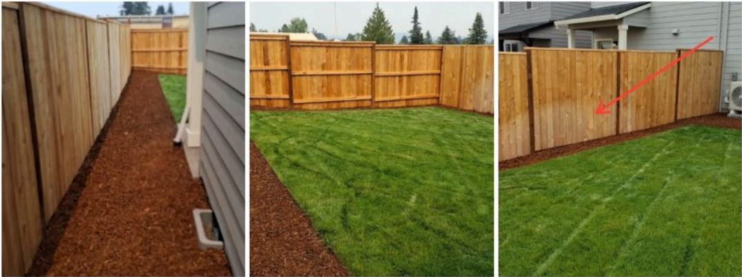
Probably a sprinkler hitting here. May want to adjust sprinkler.
